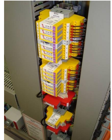
Lightning protection on CTR
