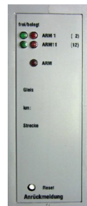
FSP evaluation unit as a train approach indicator in the signal cabin
