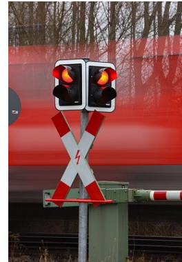
Standard level-crossing control system application
